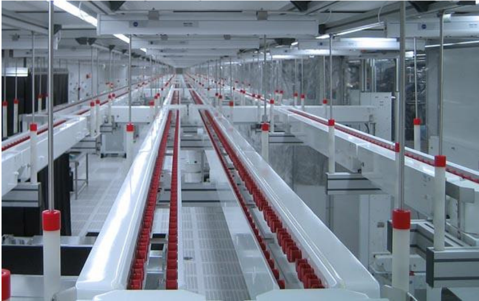
Typical Middlesex ceiling cleanroom line
